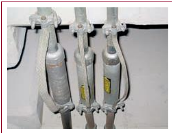
EXHIBIT 100.5 Equipment bonding jumpers installed to maintain electrical continuity around conduit expansion fittings. (Courtesy of the International Association of Electrical Inspectors)
