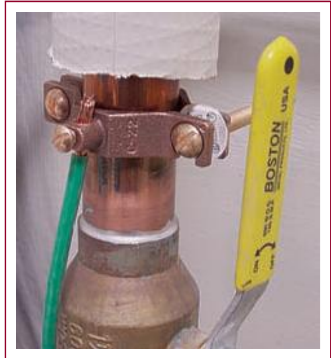
EXHIBIT 250.31 An application of a listed ground clamp.
